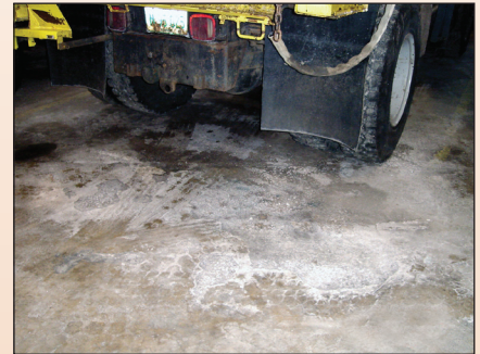
Years of salt, grease and grime had taken their toll on the concrete at Alsip Public Works.
