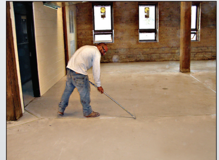
Concare, Inc. Installer Lorenzo demonstrates how fluoroelastomer is typically applied to joints.
