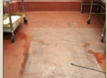
Years of spilled grease, continuous wash downs and damage from heavy cookware left the floors in the Portillo's Aurora Commissary in poor shape.
