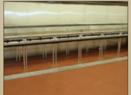
The rapid-curing GuardRight MM flooring system was installed overnight and the floor was back in service the next morning.
