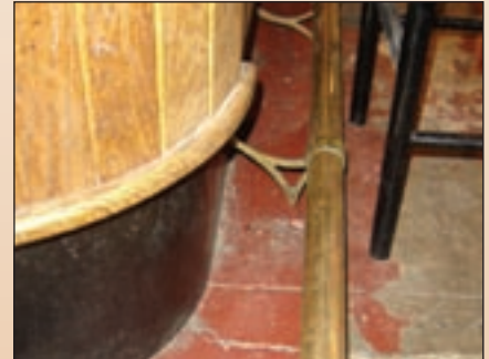
Years of high traffic made the current floor almost impossible to clean.
