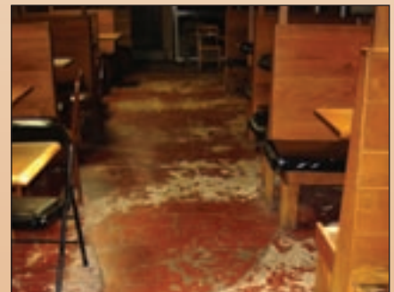
Deep cracks, odor issues and a dim, dank atmosphere led to a massive flooring renovation at The Pub.
